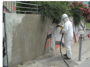
Removal of graffiti is usually done by applying the wet blasting method.
